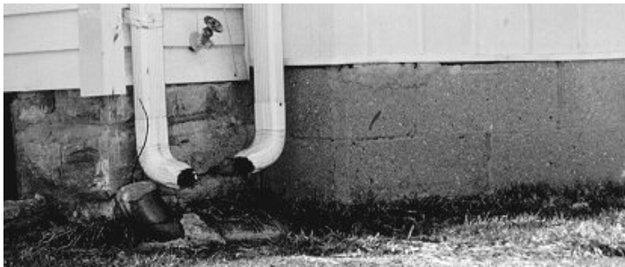
NO – Cinder block foundation (right) of new addition has not been treated to blend with the original stone foundation (left). Also, the downspouts discharge right next to the building.
