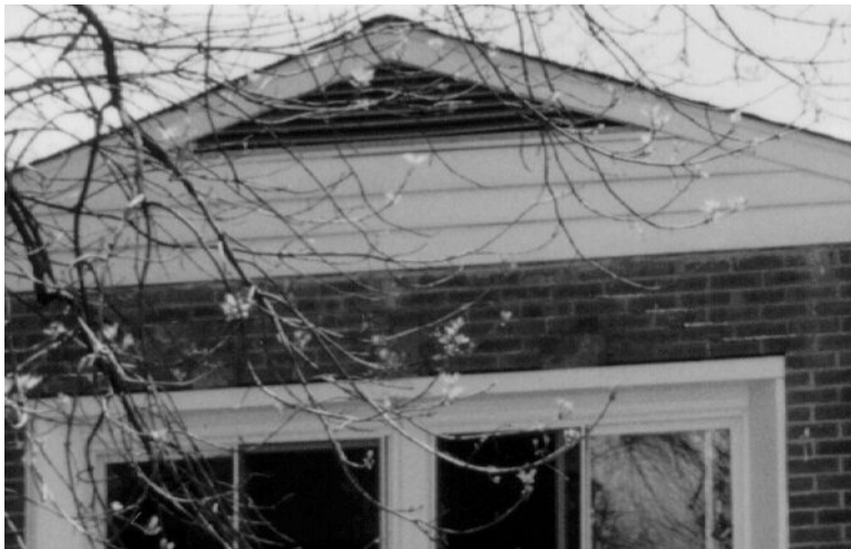
Siding such as this is inappropriate on commercial structures in the Uptown Historic District.
