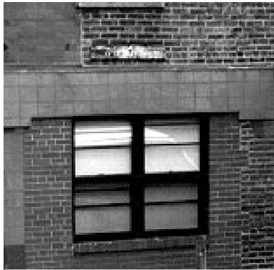
The various masonry additions to this building do not match in style, material, or
