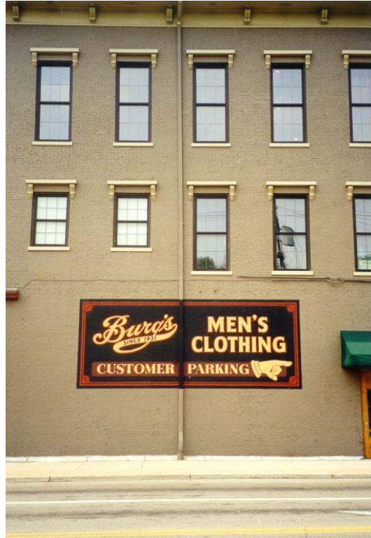
Although not located on a corner of the building, this gutter is sufficiently camouflaged by matching the painting scheme of the wall and trim.
