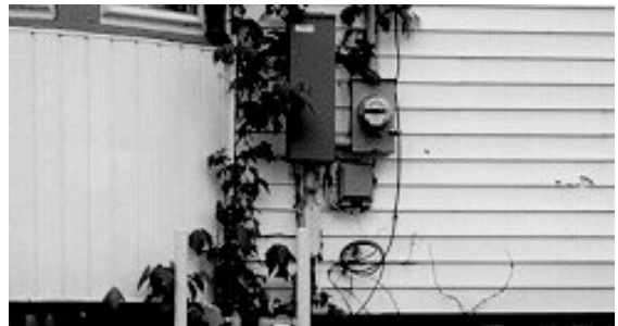
Not Like This – the bump-out window has been treated with artificial vertical siding that does not match the original horizontal wood siding to the left.
