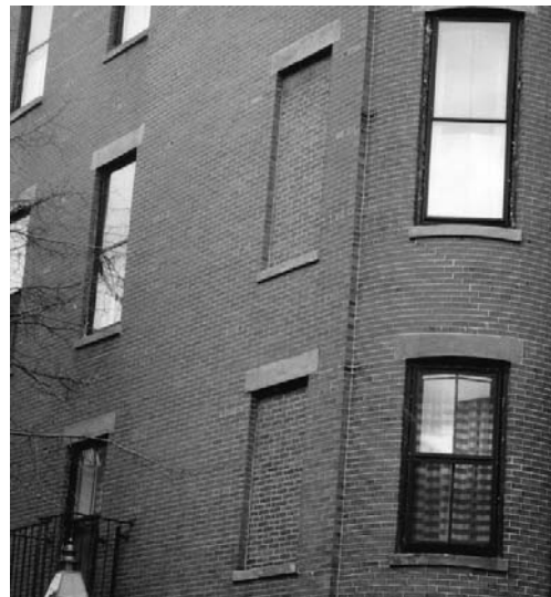
NO – In this example, the window openings have inappropriately been permanently filled with brick and the window glass removed.
