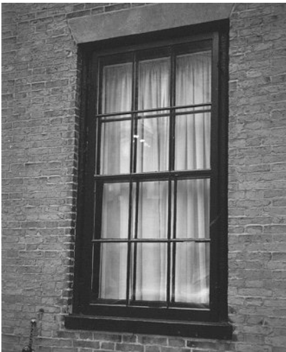
Good – Storm window exactly matches inner window.
